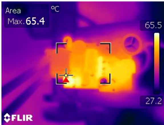
Figure 23 – With TRIAC Dimmer Connected. V_{IN} = 120 VAC, 60 Hz, 15 V LED. Load at Full Conduction. R4 was Hottest Device.
