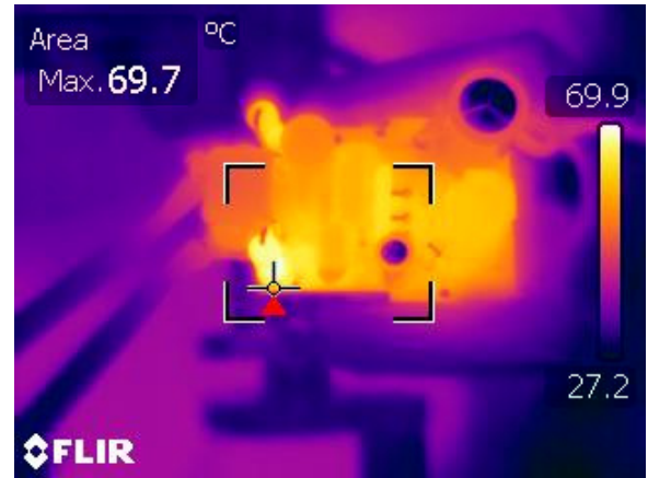
Figure 24 – With TRIAC Dimer Connected. V_{IN} = 120 VAC, 60 Hz, 15 V LED. Load at 90° Phase Conduction. R4 Damper was Hottest Device.
